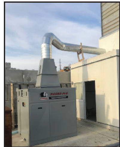
Aggre-Flo heater installed at a precast plant
