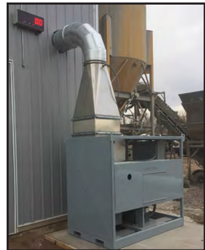
Original Aggre-Flo heater installed at ready-mix plant
